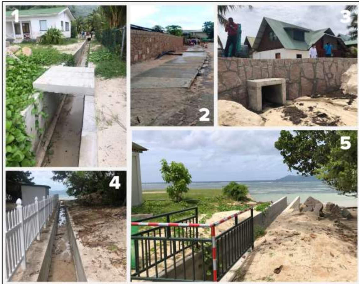
The pictures above are in line with the Outlets 1,2,3,4,5 as listed below
